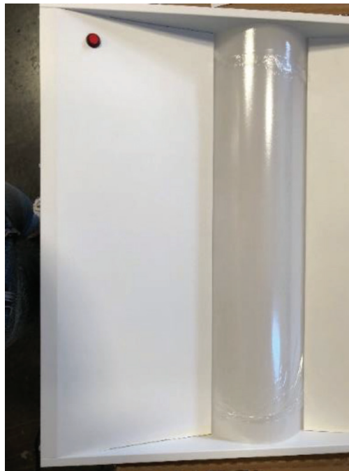
Emergency Test Button
